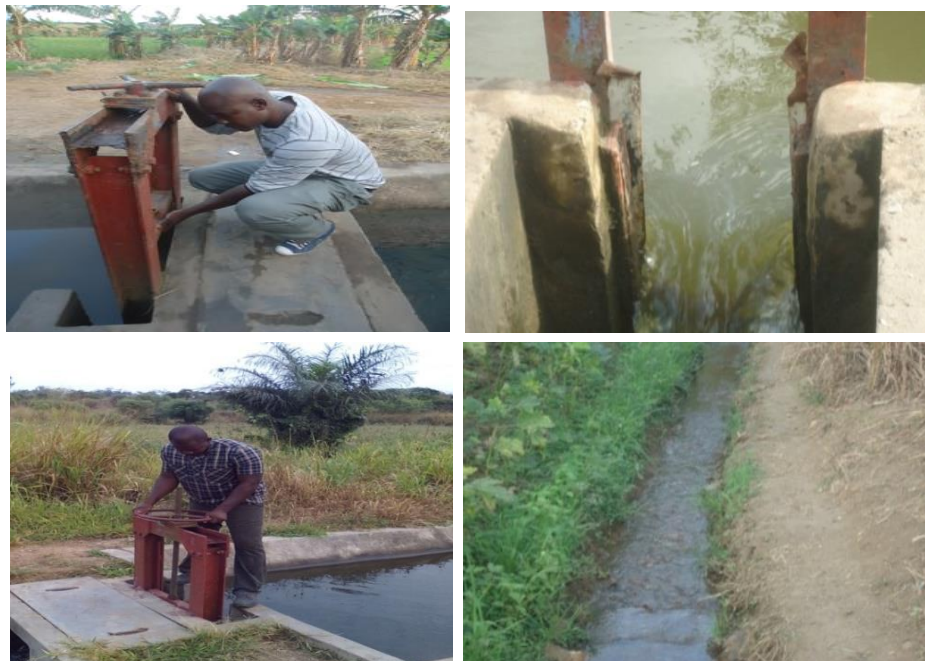
Figure 11. Some damaged check gates and an unlined tertiary canal.
